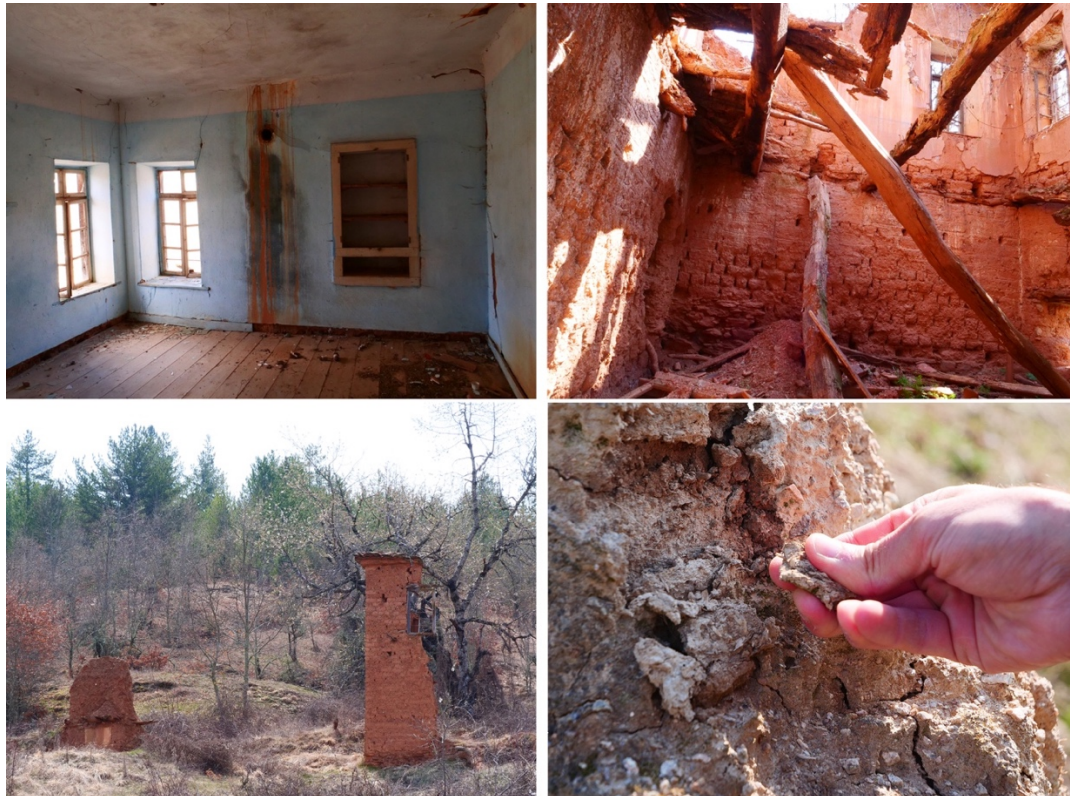
Plinth houses at the village of Ano Kranionas at various stages of decay. Photos by author, April 2019.
