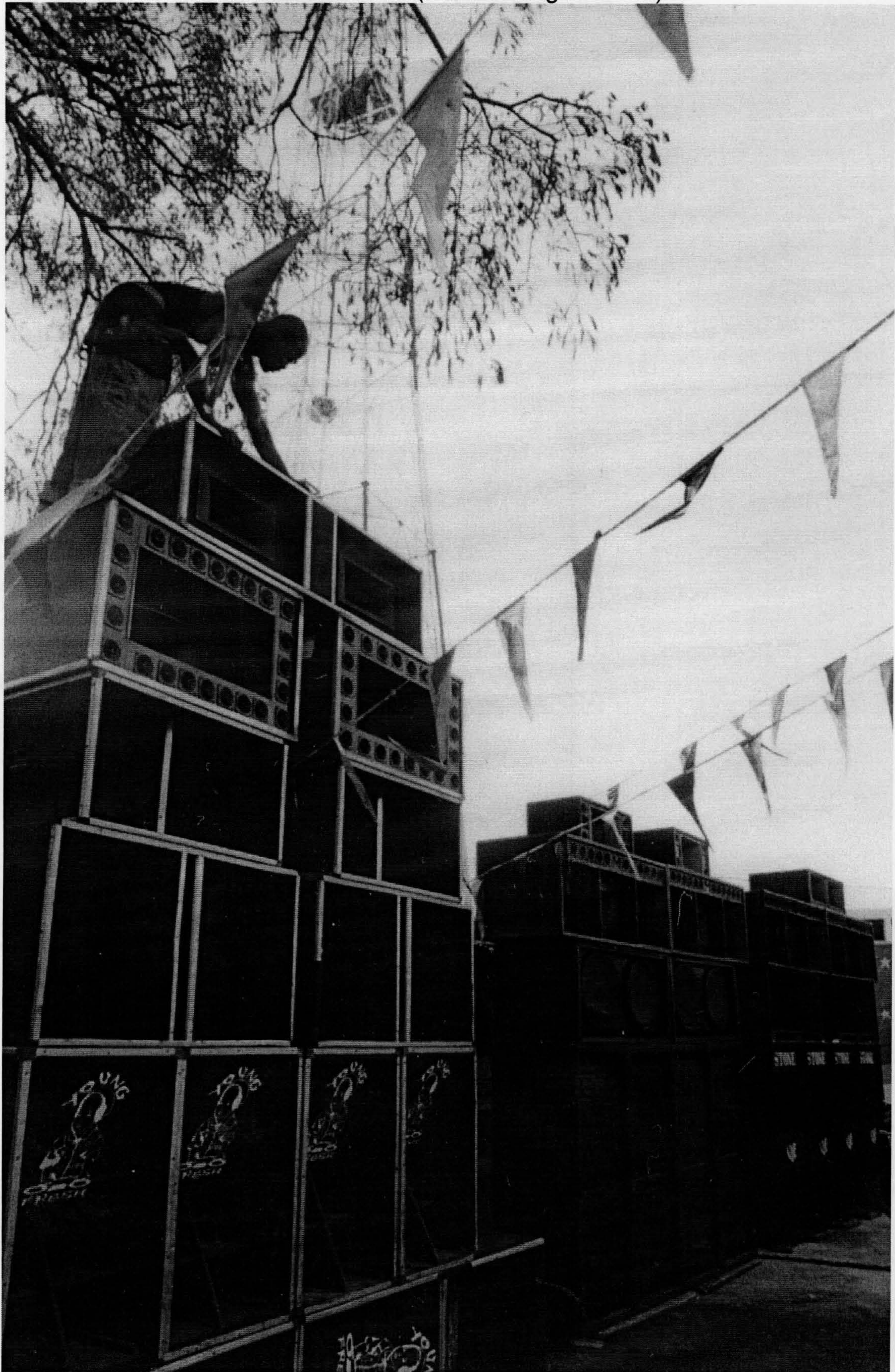
Figure 1.9 Erecting the Young Fresh Sound System speaker stacks at Skateland. Note: each sound system builds its own speaker stacks for the event, so those next to this one are those of another Sound (see also Figure A1.4).
