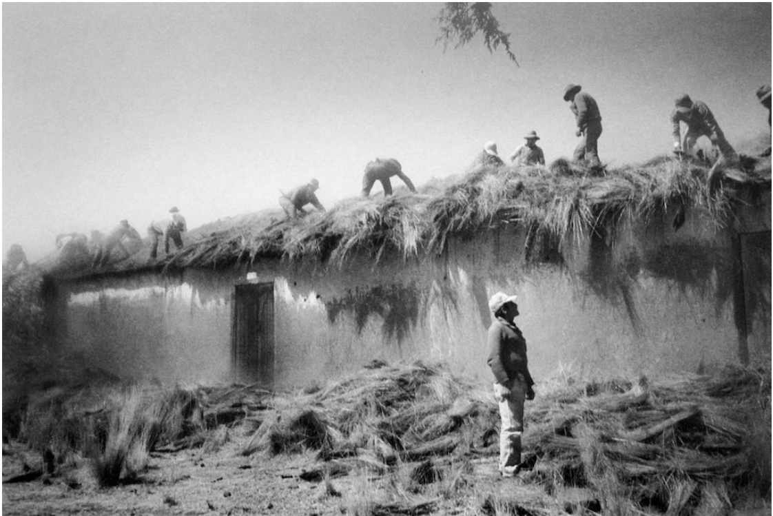
Communal work to fix the roof in the Killi Killi community Gabino Quispecondori, Ayaviri workshop, TAFOS
